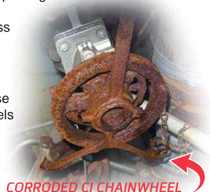
CORRODED CI CHAINWHEEL shows advantage of stainless
